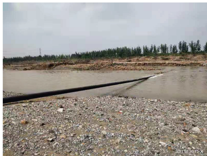
Fig. 1. Exposed pipe section after rain erosion.
