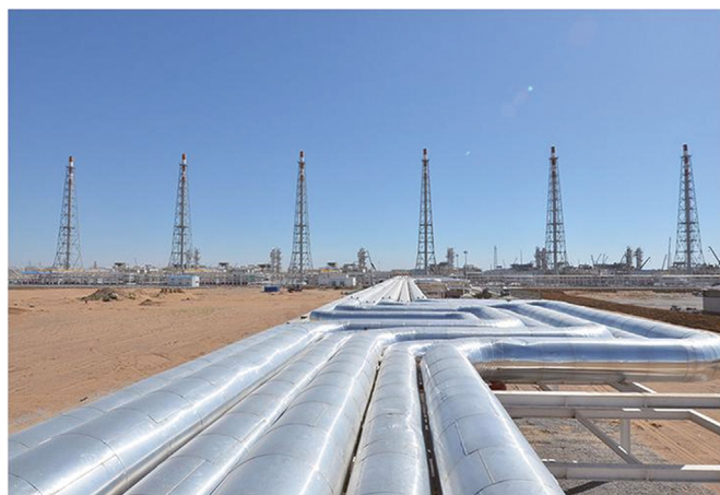
Fig. 1. Natural gas gathering pipeline.
